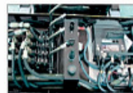
Double controllers with CANbus communication to all tube and wire
